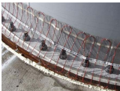
Heating elements to ensure minimum temperature
