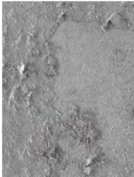
E. Improper surface preparation of existing coating
