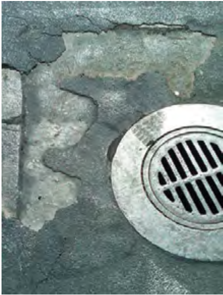
A. Improper concrete surface preparation
