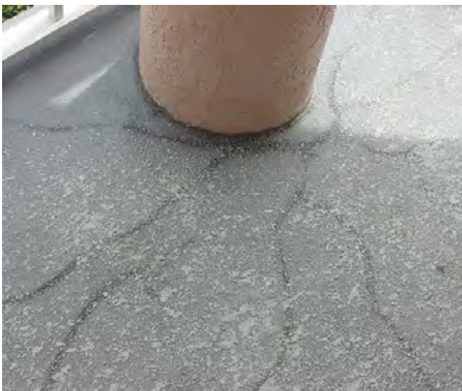
B. Improper sealant chemistry
