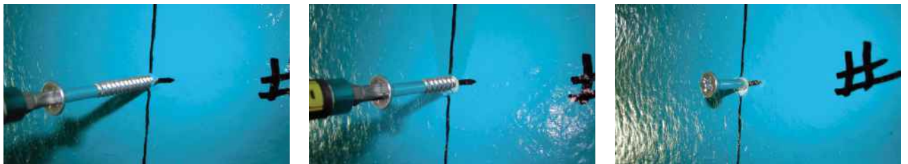
Air barrier leak caused by screw penetration
