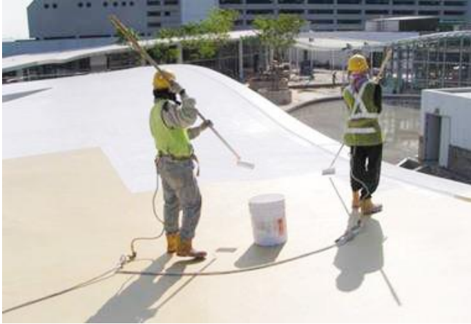
Application of waterproofing on roof of VivoCity (Singapore). Photo courtesy of Mapletree Investments Singapore.
