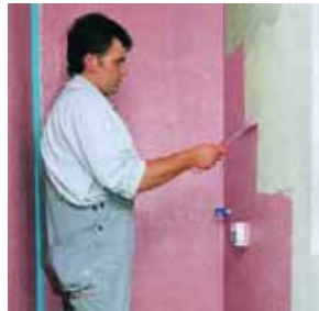
2. Apply undiluted MasterTile WP 668 (red) to the substrate as a first protective coating to cover its entire surface.
