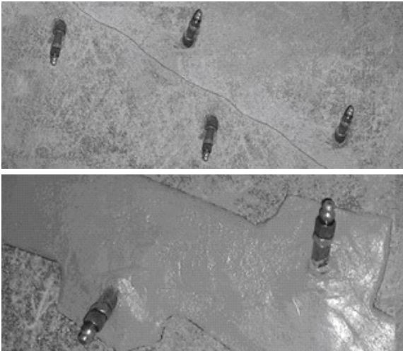
Figure 1. Socket type nipples placed around the crack and sealed with proper MasterBrace epoxy adhesive.
