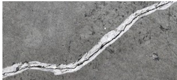
Figure 2. V shaped groove opened on the crack.
