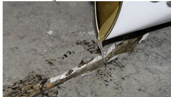
Figure 4. Pouring MasterInject 1360 directly into the V shaped groove opened on the crack.
