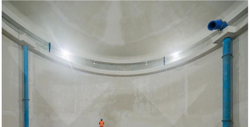
Our reference project in Feluy, Belgium: new water tower (Designed by IDEA)
