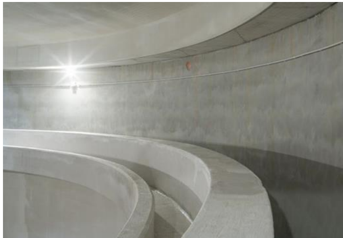
Our reference project in Feluy, Belgium: new water tower (Designed by IDEA)
