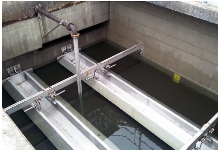
Our reference in West Wales (United Kingdom): Water Treatment Works
