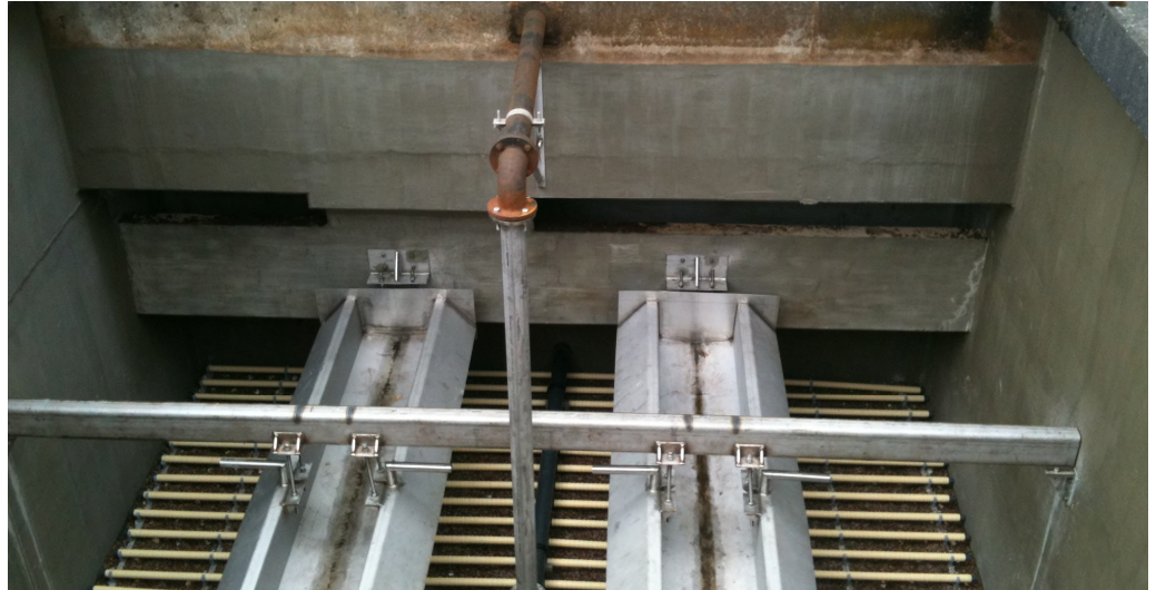
Our reference in West Wales (United Kingdom): Water Treatment Works
