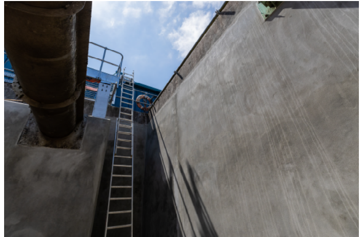
Our reference in Northern Ireland (United Kingdom): Water Treatment Works
