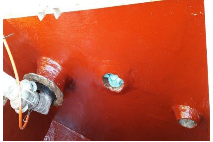
Our reference in Suffolk (United Kingdom): Waste Water Inlet Chamber
