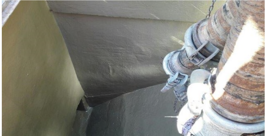
Our reference in Suffolk (United Kingdom): Wastewater Inlet Chamber
