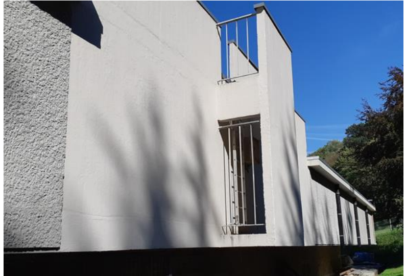
Our reference project in Lustin (Belgium): the Vivaqua-Tailfer sludge treatment building after remediation
