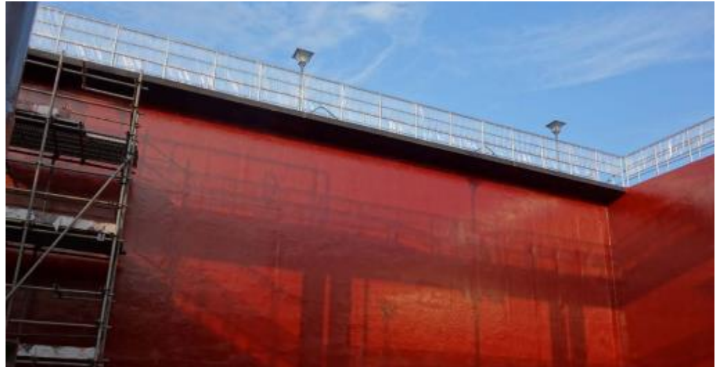
Our reference in Shanghai (China): inside of an aeration tank, part of the new integrated water and wastewater treatment services for SCIP
