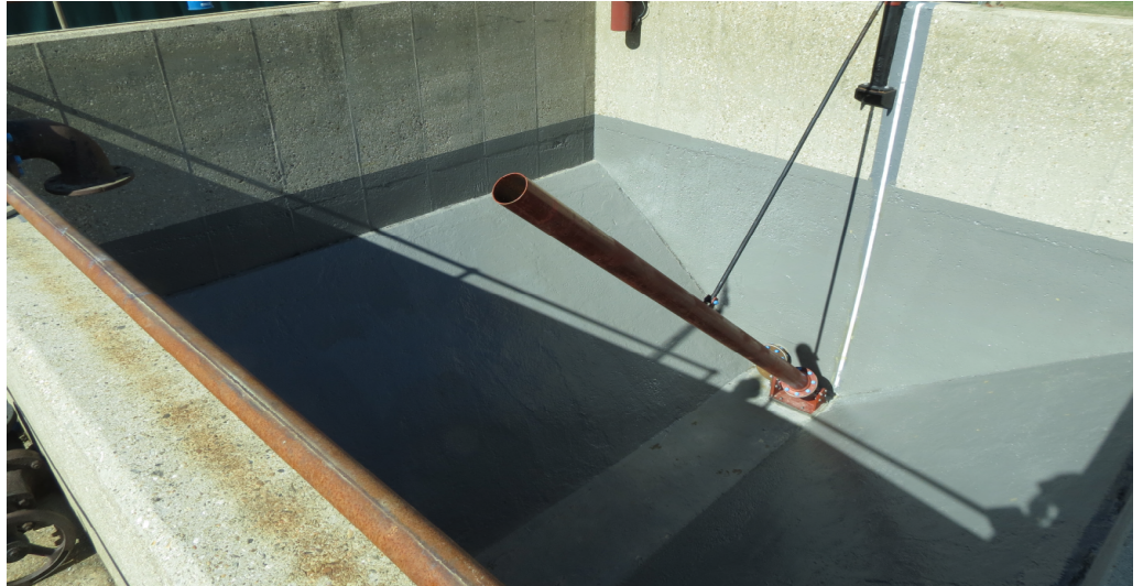
Our reference in Southampton (United Kingdom): Sewage Water Treatment Works
