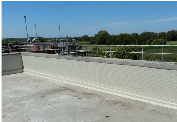
Our reference in Glastonbury (United Kingdom): Sewage Treatment Works
