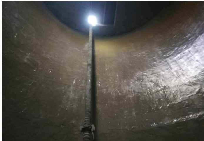
Our reference in Wisbech (United Kingdom): Sewage Pumping Station Shaft
