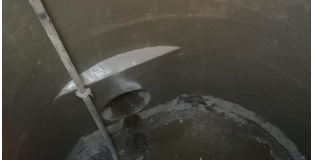
Our reference in Wisbech (United Kingdom): Sewage Pumping Station Shaft
