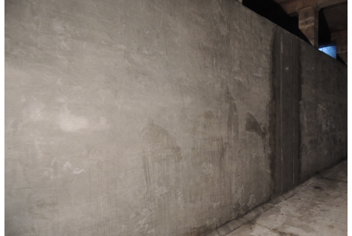
Our reference in Warwick (United Kingdom): Service Reservoir
