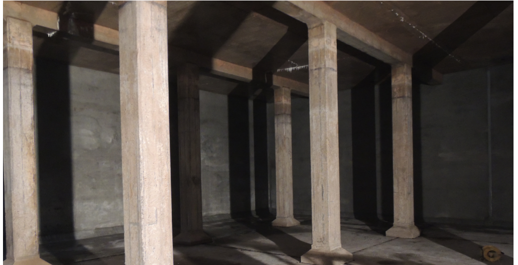
Our reference in Warwick (United Kingdom): Service Reservoir
