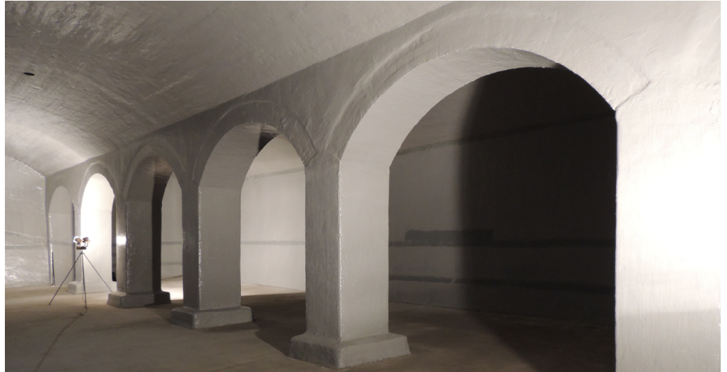
Our reference in Surrey (United Kingdom): Service Reservoir
