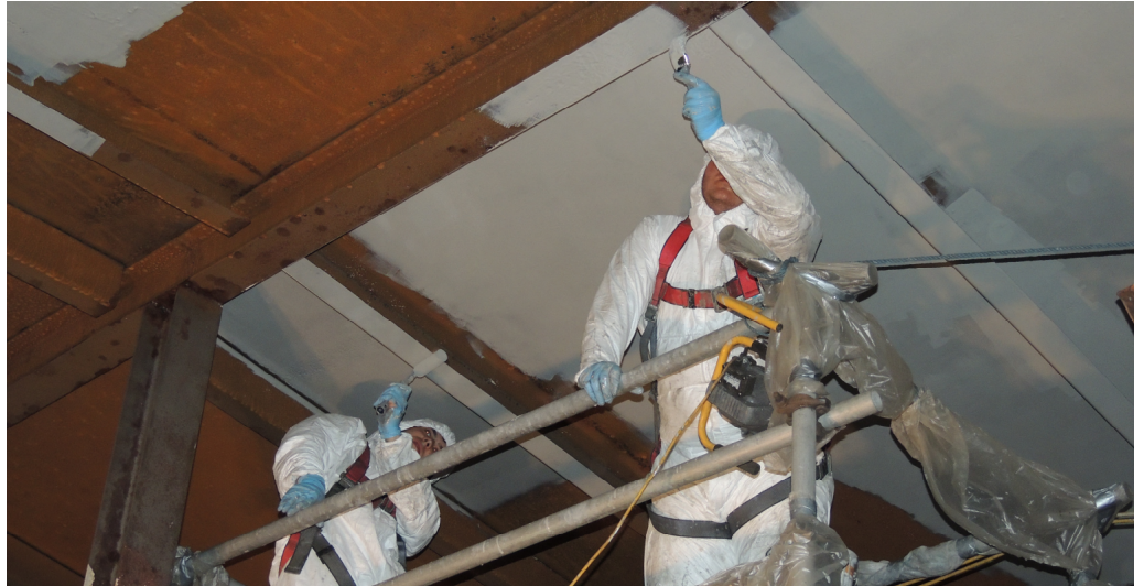
Our reference in East Sussex (United Kingdom): Service Reservoir
