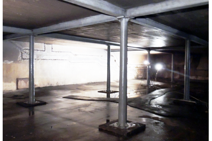
Our reference in Kent (United Kingdom): Service Reservoir
