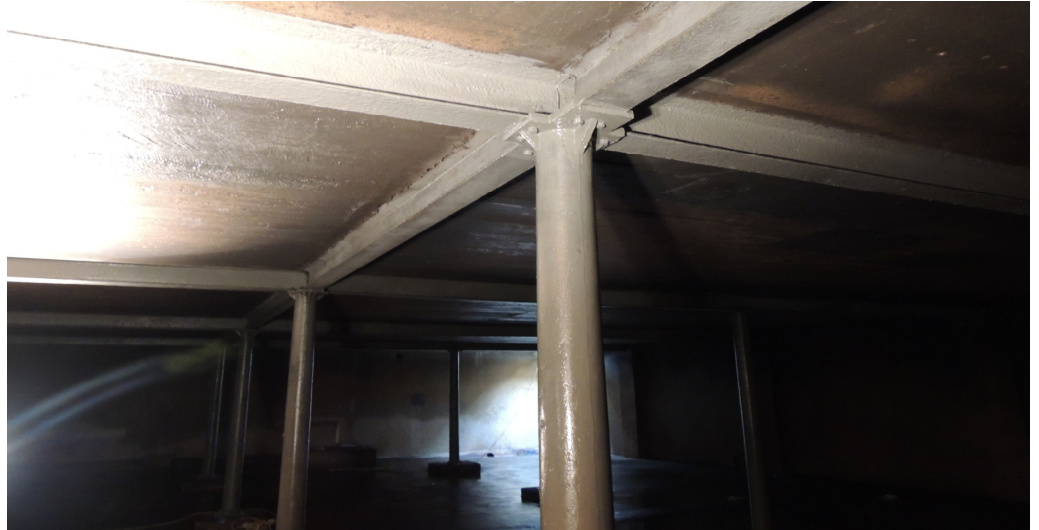
Our reference in Kent (United Kingdom): Service Reservoir
