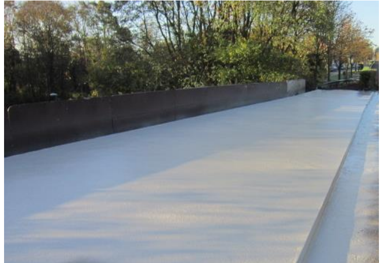
Our reference in Leuven (Belgium): Ring road Leuven: Side walk roads waterproofing
