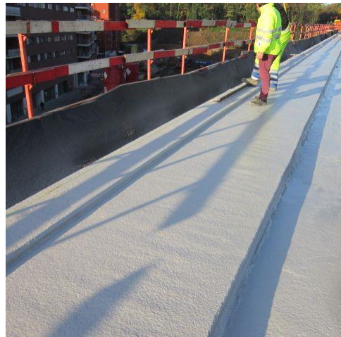
Our reference in Leuven (Belgium): Ring road Leuven: Side walk roads waterproofing
