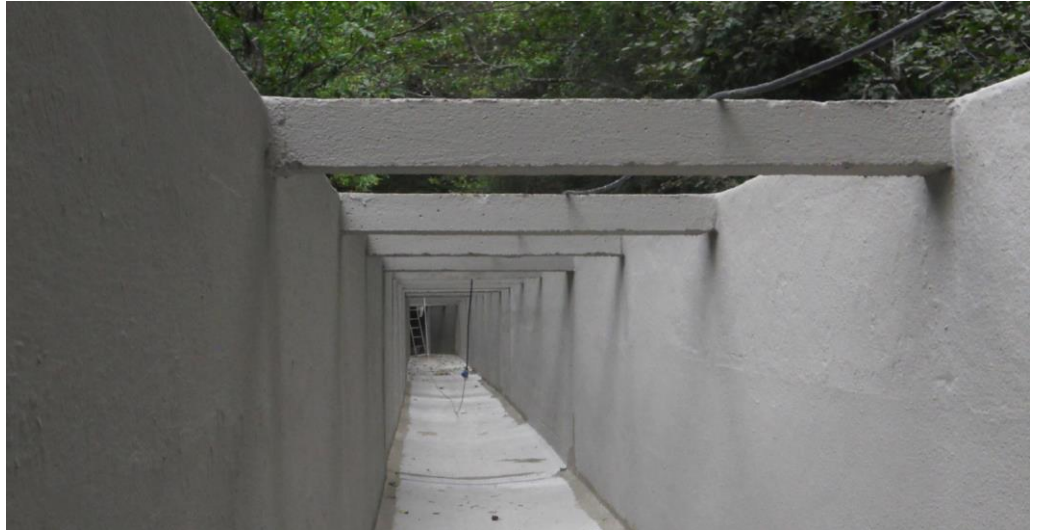
Our reference in Garfagnana, Lucca (Italy): ENEL Hydroelectric station
