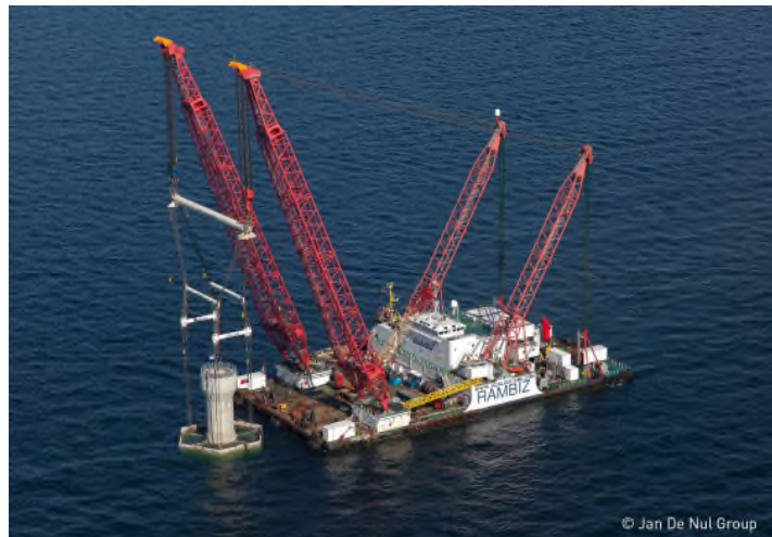
Our reference in the Baltic Sea(Sweden): Kårehamn Offshore Windfarm
