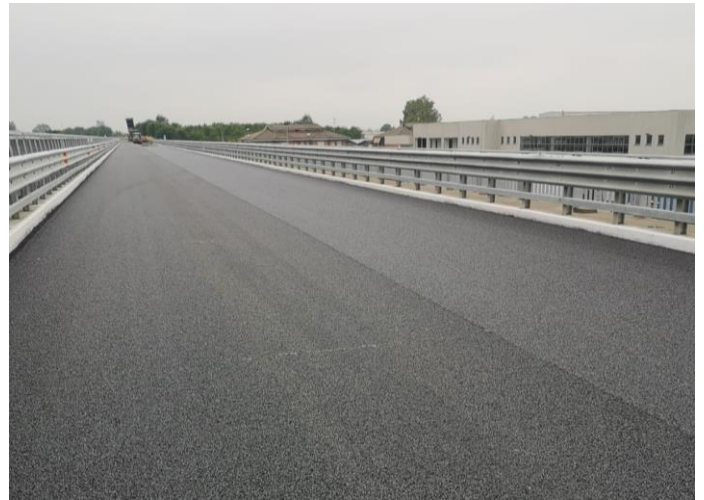
Our reference project in Fossano (Italy): Waterproofing of viaduct deck with MasterSeal 6100 FX
