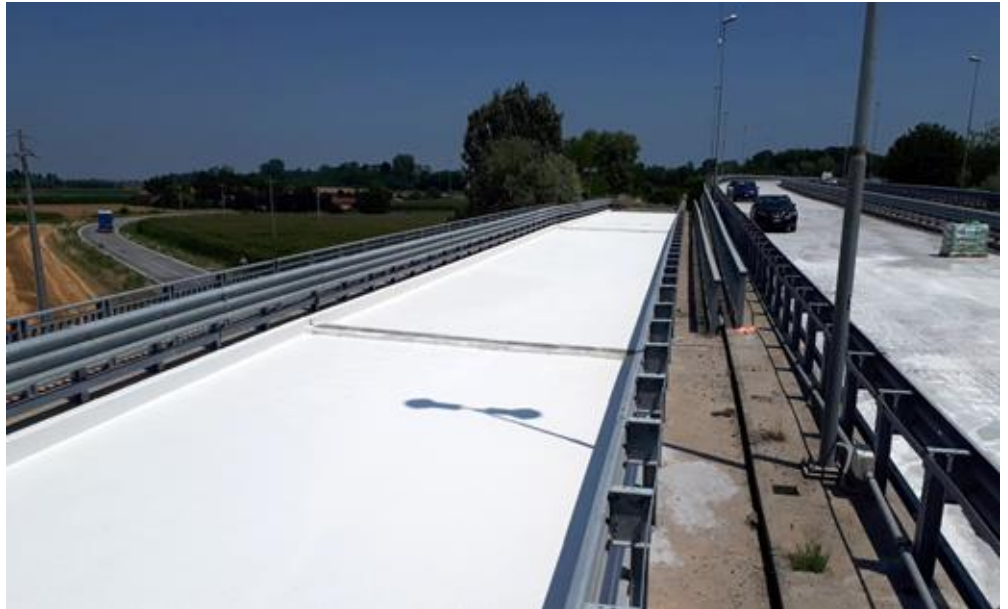
Our reference project in Fossano (Italy): Waterproofing of viaduct deck with MasterSeal 6100 FX
