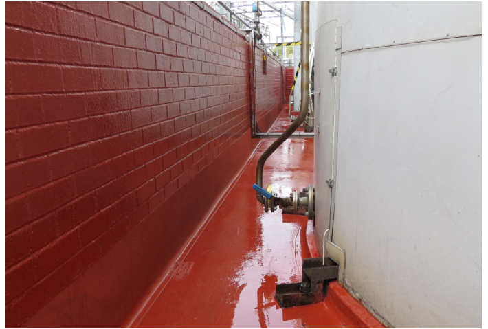
Our reference in Bradford (United Kingdom): Chemical Plant Bund
