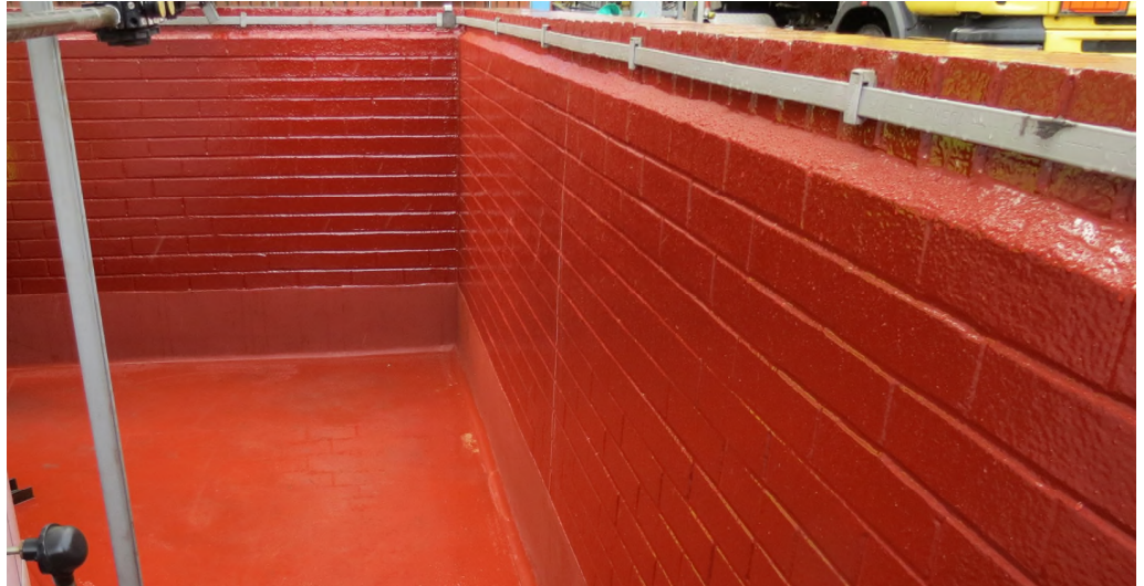
Our reference in Bradford (United Kingdom): Chemical Plant Bund
