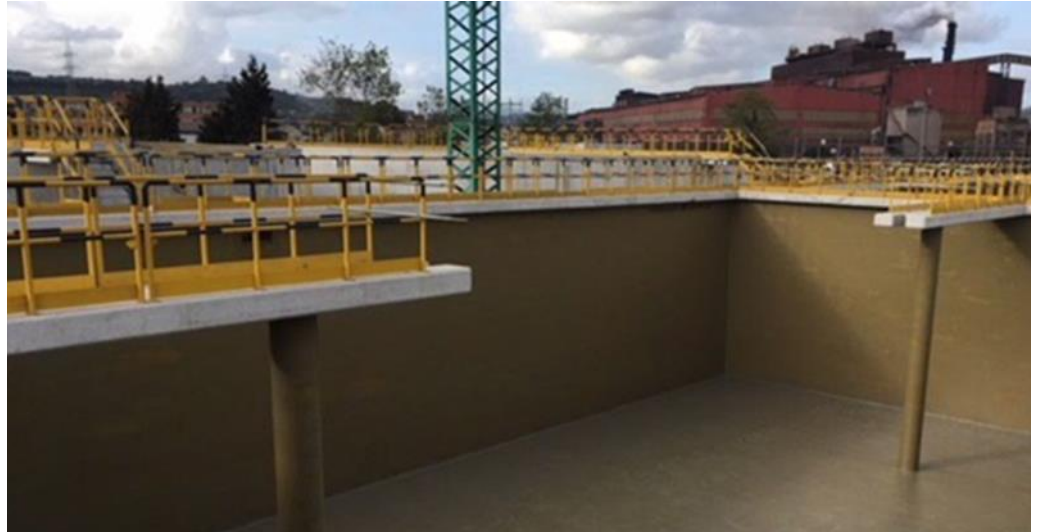
Chemical protection for reinforced concrete tanks using MasterSeal 7000 CR system (Asturias Spain)
