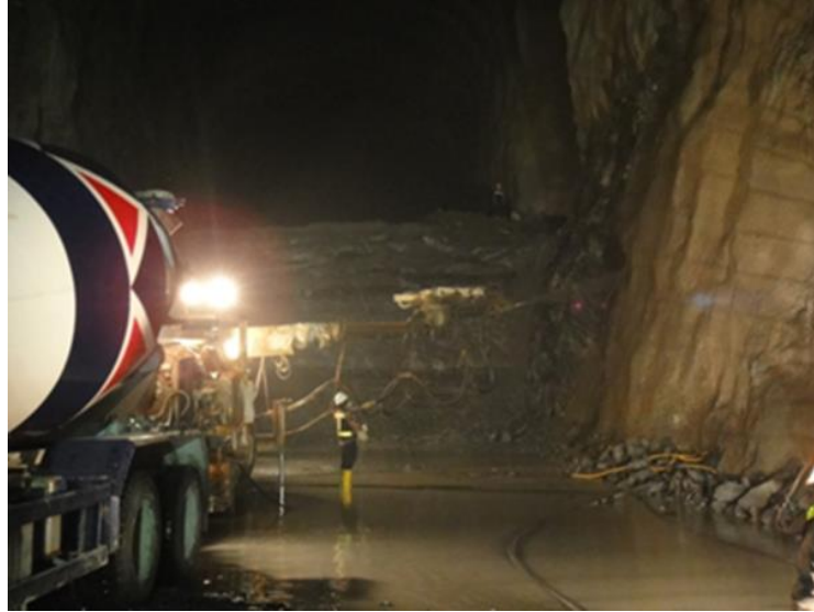
Our reference of Jurong Rock Cavern Phase 1 (Singapore). Photo courtesy of JTC Corporation.
