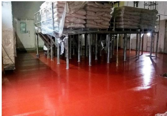
Sugar dumping area applied with Ucrete UD 200
