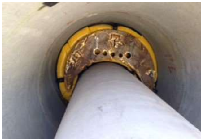
Mock-up of the inflatable bags after filling with precision grout sealing the tunnel annulus
