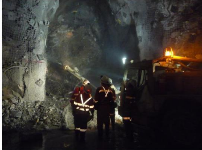
Sprayed concrete (shotcrete) trial at Kencana and Toguraci underground mine, Gosowong gold project
