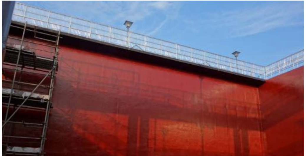
Our reference in Shanghai (China): inside of an aeration tank, part of the new integrated water and wastewater treatment services for SCIP
