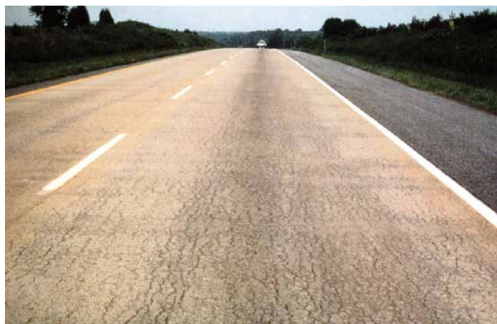
Figure 1. ASR-Induced Map Cracking in Pavement
